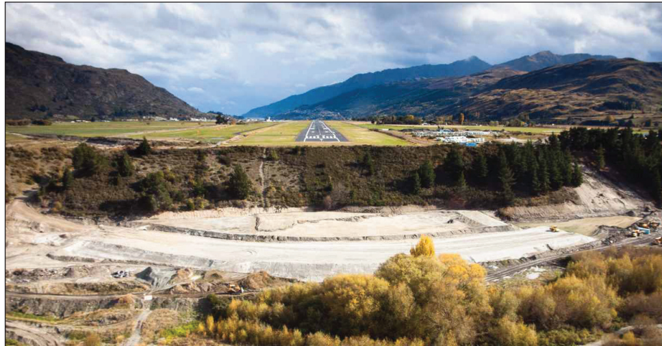
QUEENSTOWN AIRPORT: The development involves excavating one million cubic metres of spoil to be used for a runway extension
