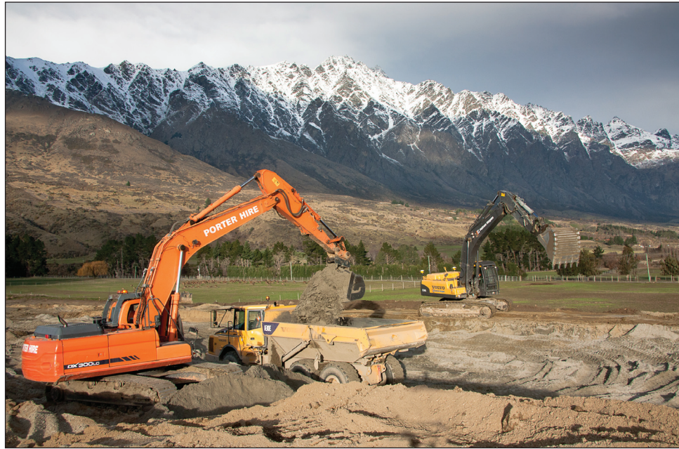
WORK STARTS: Porter Group is digging away at its Remarkables Park project
